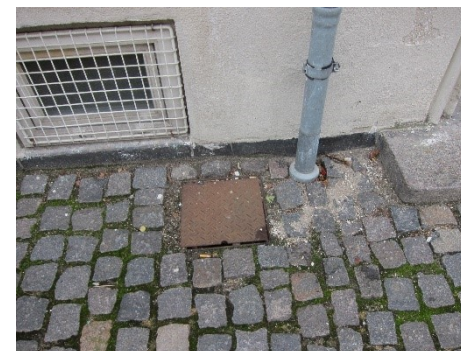
Tagbrønd mod gade
